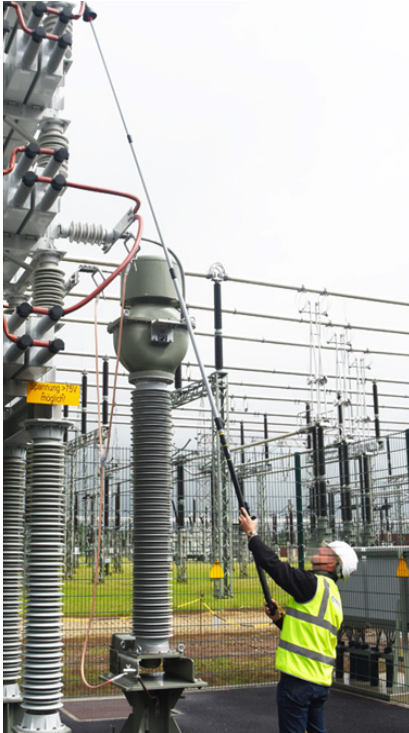
Test at a 36 kV compensation system
