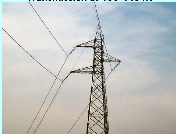
Transmission at 130-145 kV
