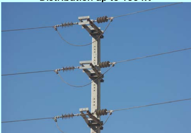
Distribution up to 100 kV
