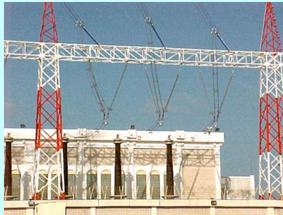
Transmission at 400 Kv
